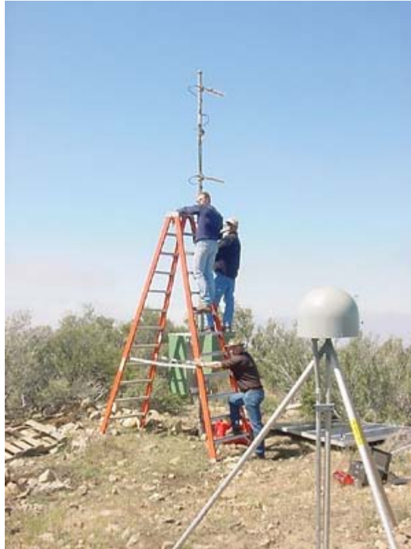
Glen Offield, Robert Deal and Craig Whaley install radio repeater antennas on Modjeska Peak.
